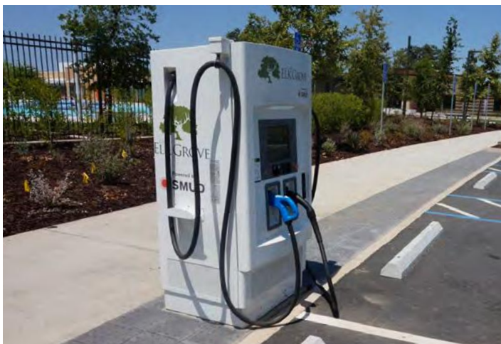
EV charging stations in Elk Grove
