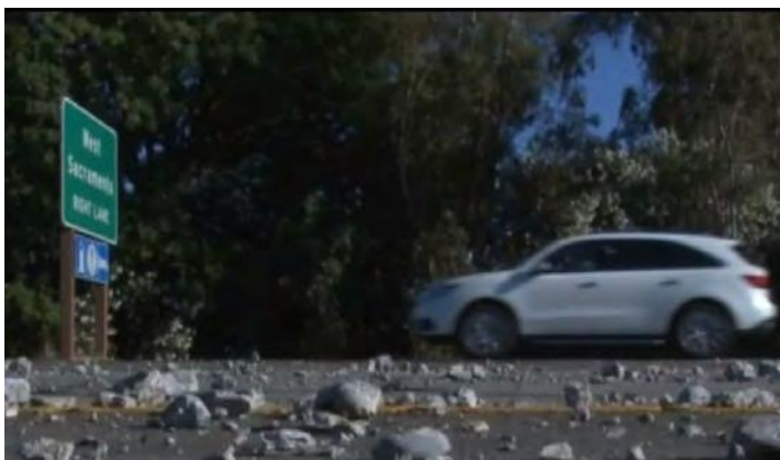
Extreme heat events can result in concrete roadway blowouts in which the pavement expands and can buckle or explode. Highway 50 in West Sacramento experienced blowouts from extreme heat in 2017 (shown above).
